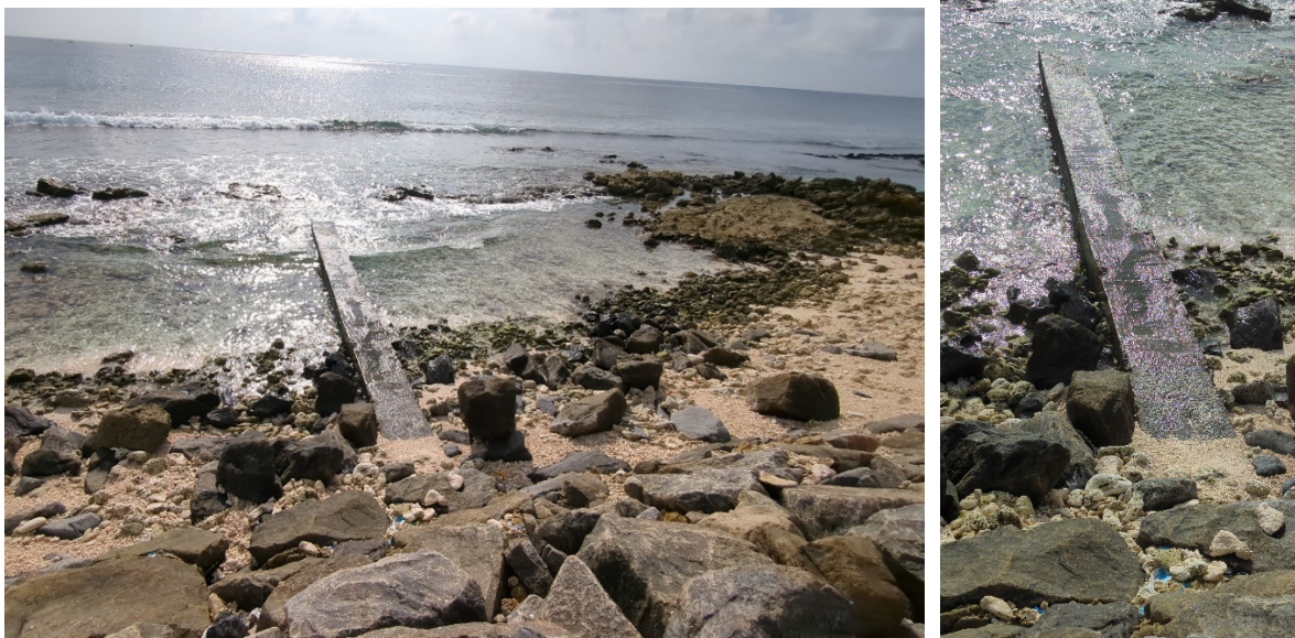
Figure 27: Submarine communications cable entering the island, under the revetment
